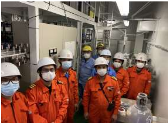
Experts and crew in the CO2 capture plant
